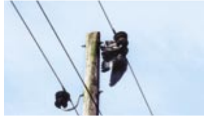
Wood poles can become a hazard in wet weather as they lose their insulating capacity.
