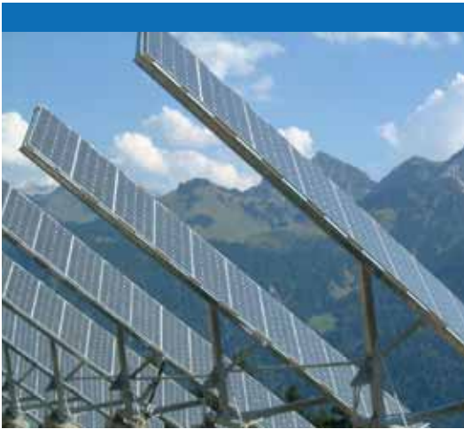
Photovoltaics at Blonz (© Gr. Walsertal BR)
