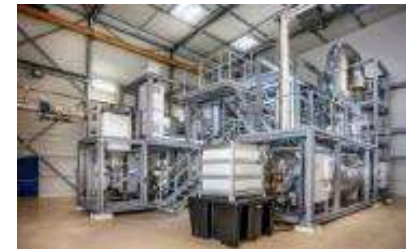
Off Gas Treatment (OGT)
